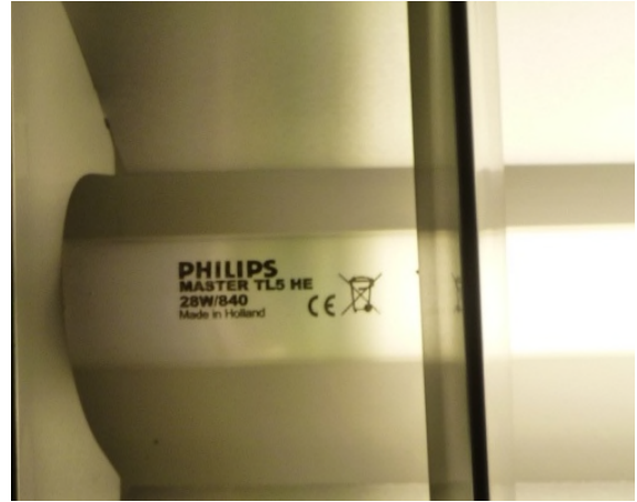
Lamp wattage clearly visible
