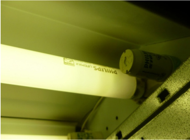
Lamp facing the wrong way, wattage not visible
