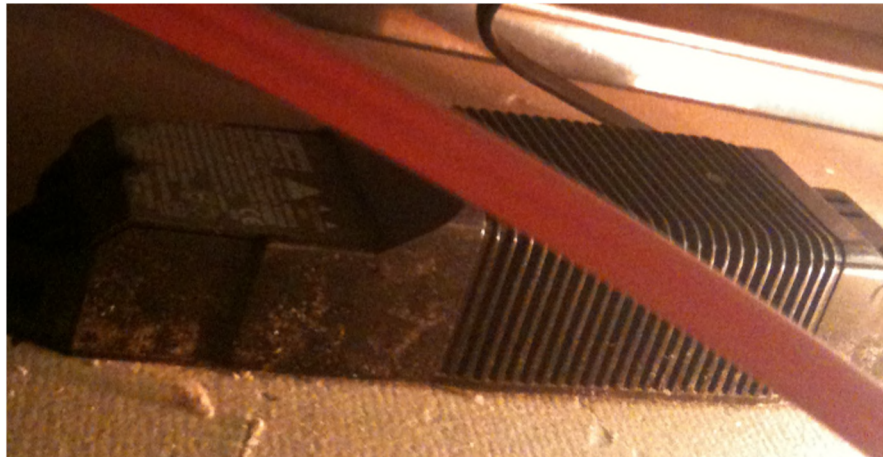
Figure 5: Magnetic transformer in ceiling space
