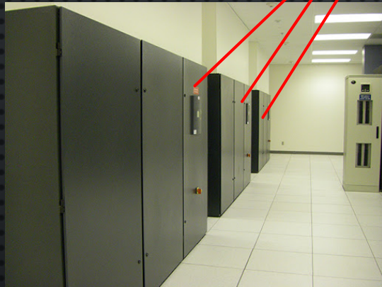
Individual CRAC Units
